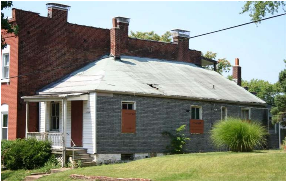
FRONT AND NORTH ELEVATIONS – SHOWING ROOF CONDITION
