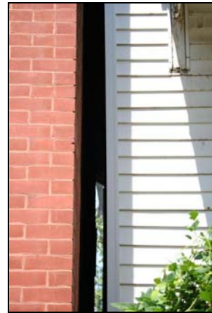
SPACE BETWEEN ADJACENT BUILDING, ATTACHED AT ROOFLINE
